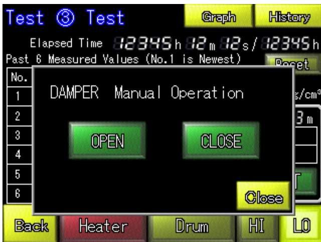
Fig.3.3c Test③ (SA Damper Manual Operation)
